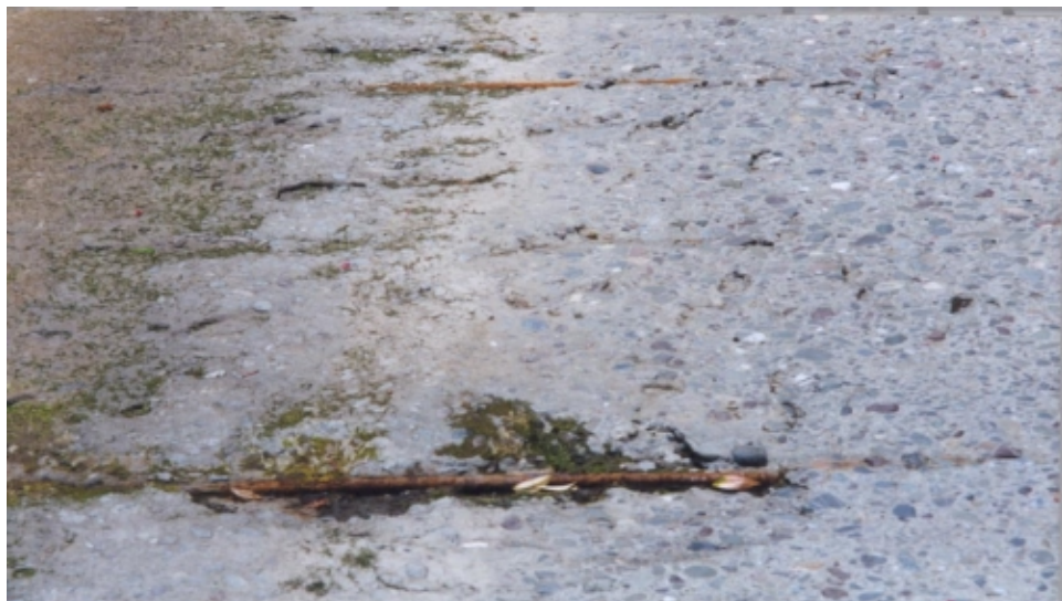
Figure 5. Degraded channel invert
